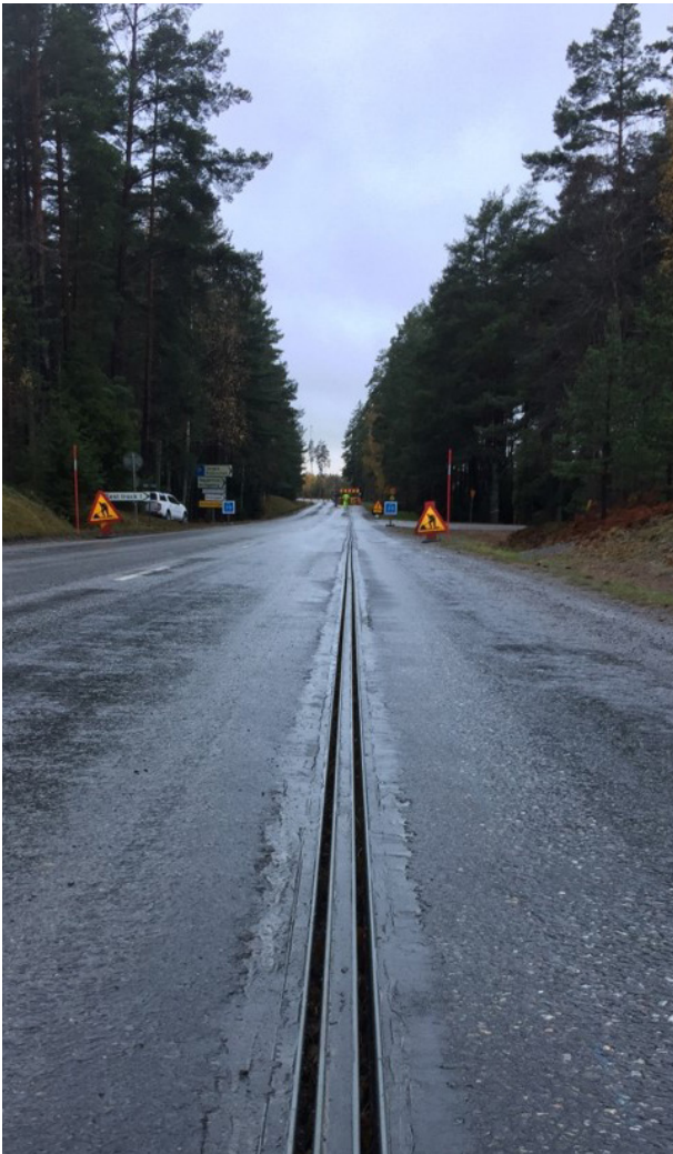
Photo 1: Elways rail fitted to the Arlanda e-Road pilot project in Sweden. Source: Elways.
