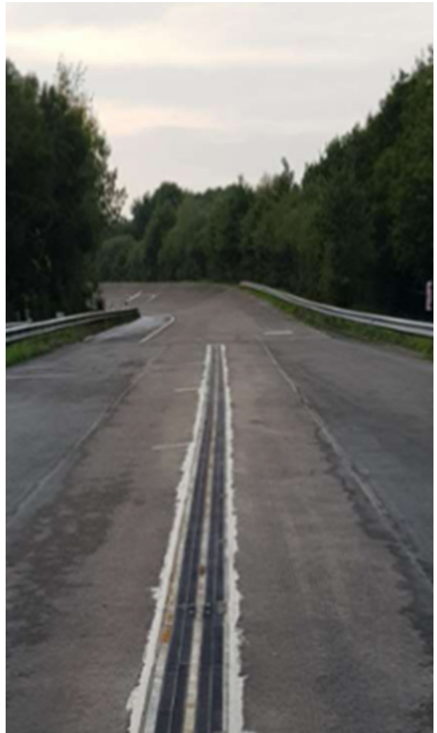
Photo 2: Alstom system with double rail integrated into the road. Source: Alstom
